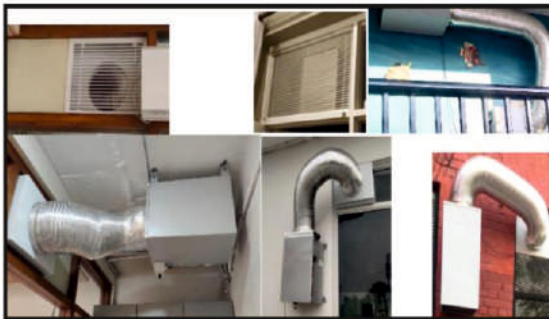
Clean Air & HVAC Solution
